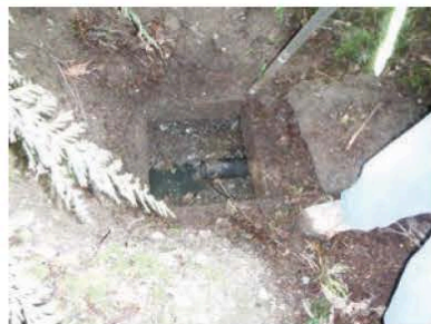
According to Alan Chapin, this tank received an OK from a previous point-of-sale inspection. The inlet baffle was missing and an inadequate 3-inch ABS pipe was used.
