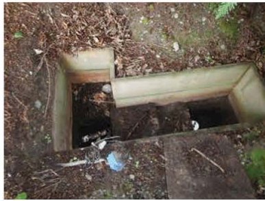
During a follow-up inspection, Alan Chapin found an interior electrical box used outdoors and no cover over a makeshift wooden frame exposing tank access lids. (Photos courtesy of Alan Chapin)
