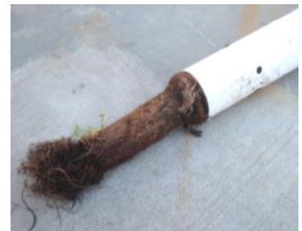
Root intrusion into drainfield. Roots filled the piping and caused the drainfield to prematurely fail.
