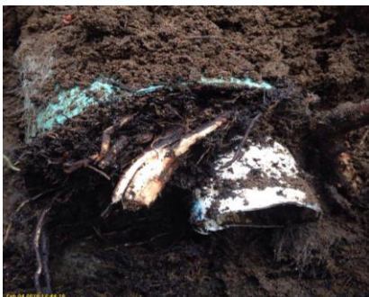
Severe root damage to drainfield, we were able to pull most roots out and jet the rest of the lines to prolong the drainfield life.
