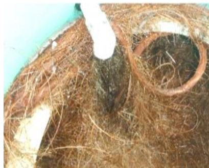
Root intrusion into tank. Found too late and caused riser damage along with other expensive repairs.
